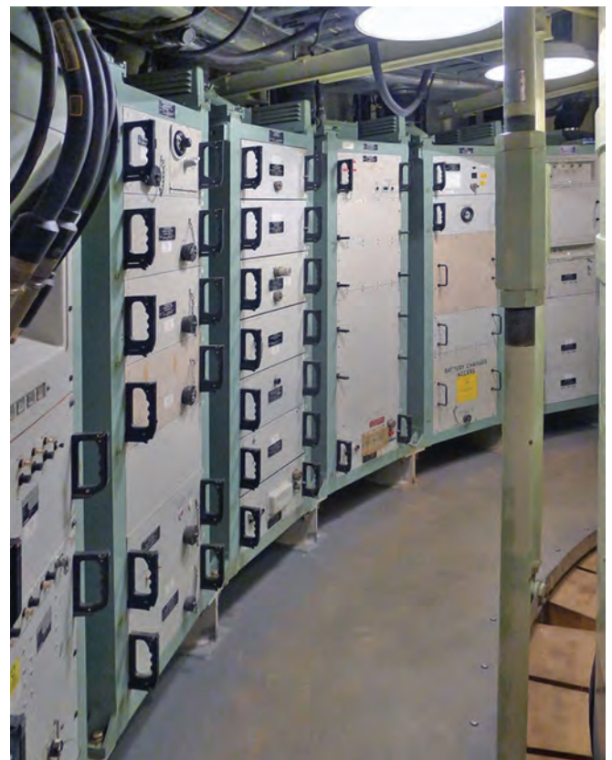
Silo equipment area level 1. Racks of launch support equipment are housed on a shock mounted platform
